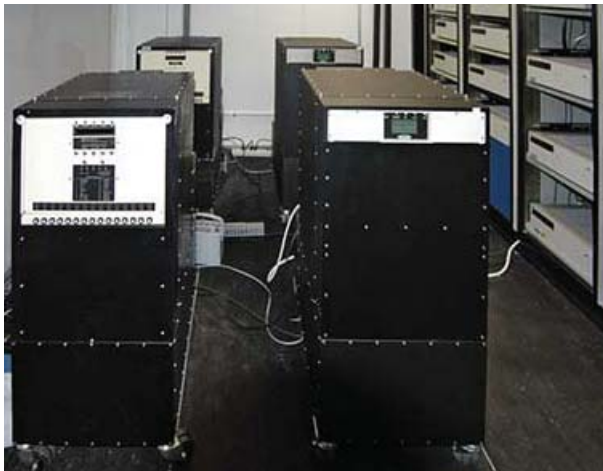
FIGURE 10 one of the USNO clock vaults containing Symmetricon's masers and cesium instruments
